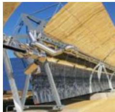
Parabolic trough application
